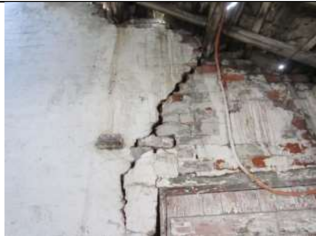
Photo 32: Crack at interior of Outbuilding 1, Section 1b
