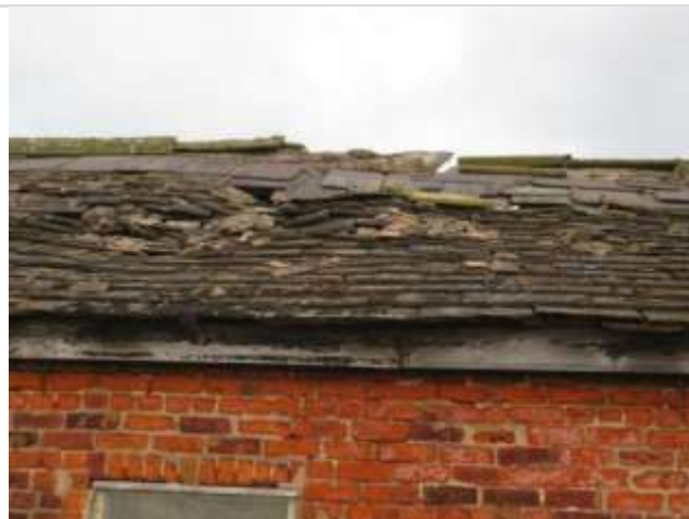
Photo 30: Collapsed roof at Outbuilding 1, Section 1b
