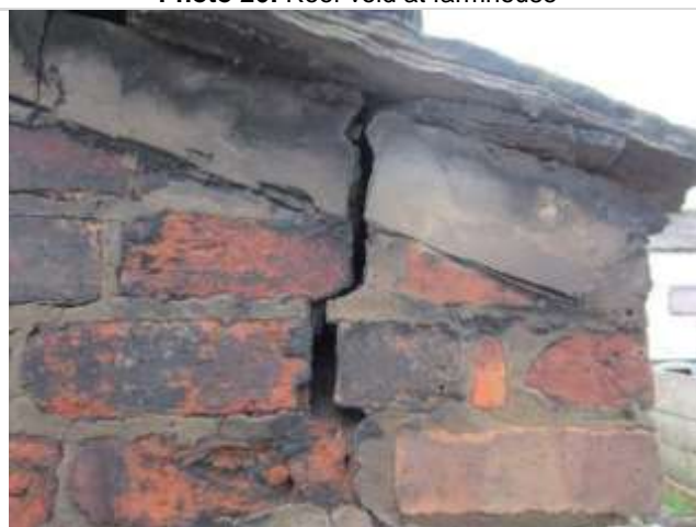
Photo 28: Crack at northern elevation of Outbuilding 1, Section 1a
