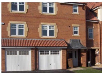
Lack of habitable room windows at ground floor.
