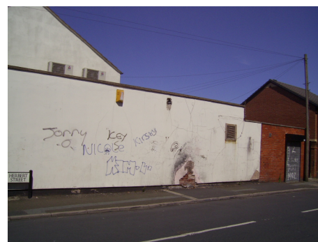
Poor materials are prone to vandalism.
